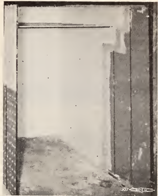
Photo No. 4. Corridor Walls and Ceiling showing Insulated Suspended Ceiling and Insulated Outside Wall. Also Rocklath Air Duct in Corridor. (See Detail No. 4.)
